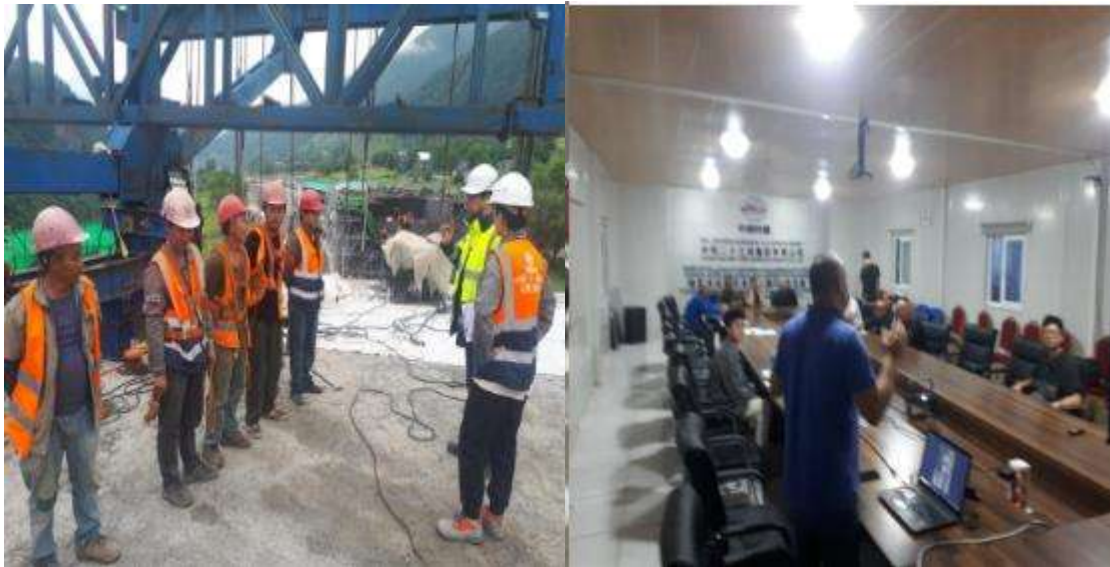
Figure 35: Toolbox Talks with Crew and Working at Heights Trainings at Lot 2 (July 2024)
